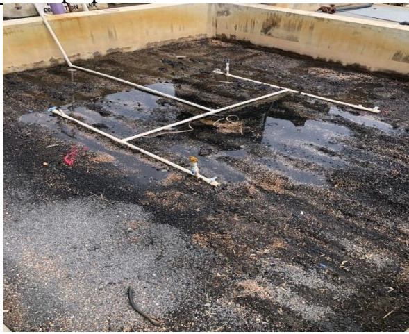
Sand-gravel & Carbon filter bed
