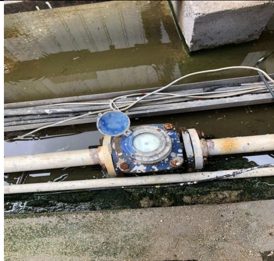
RO permeate flow meter
