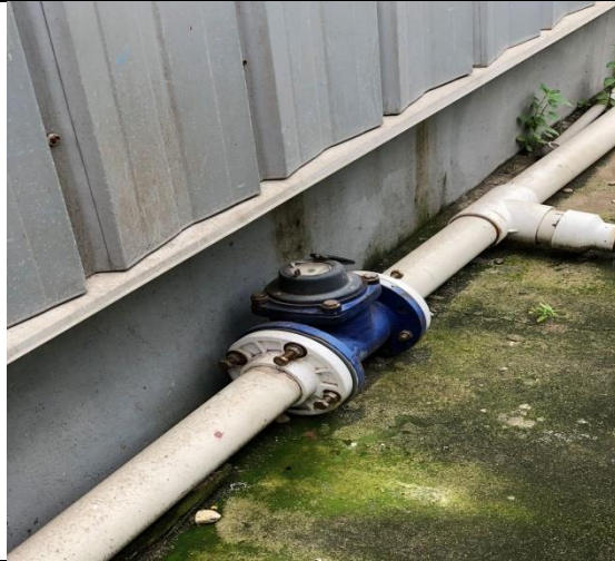
Flow meter on DM water supply line
