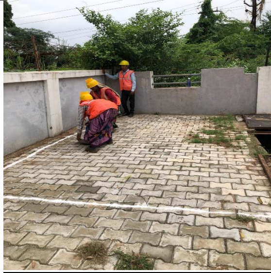
Location where unit will construct cabin for provision of RTOM, auto sampler, IOT, 3-way valve, flow meter etc as per VECL directions
