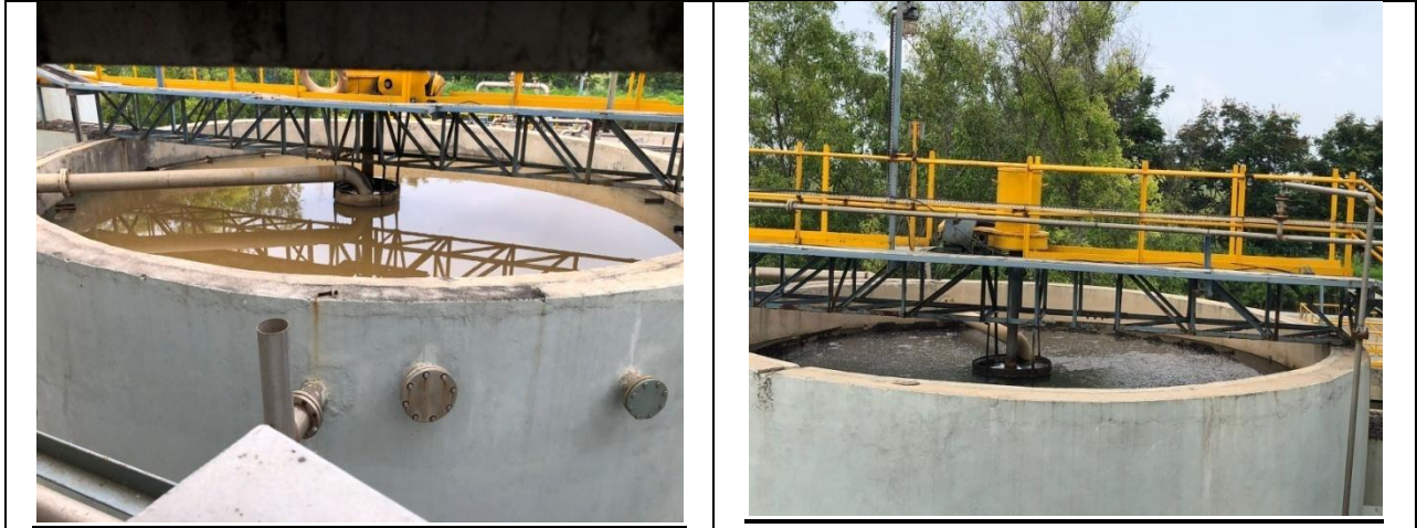
Operational condition of Primary Clarifier and secondary clarifier was not satisfactory
