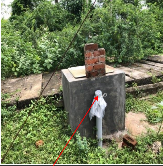
Discharge pipeline for disposal of effluent into VECL is observed disconnected.
